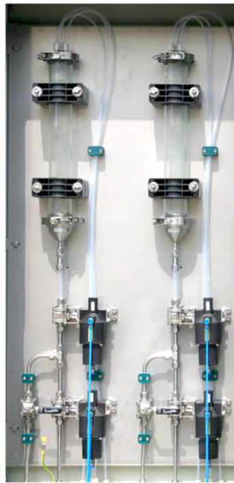
Customized preconditioning system on site
